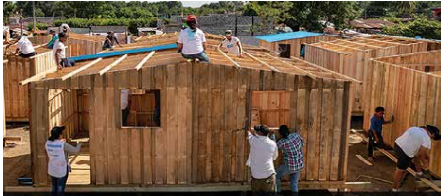
Construction continues on CRS-supported transitional shelters for community members displaced by the volcanic eruption in Guatemala. Photo by Ivan Palma/CRS
